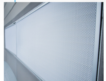
Back of unit. H14 HEPA filter.
